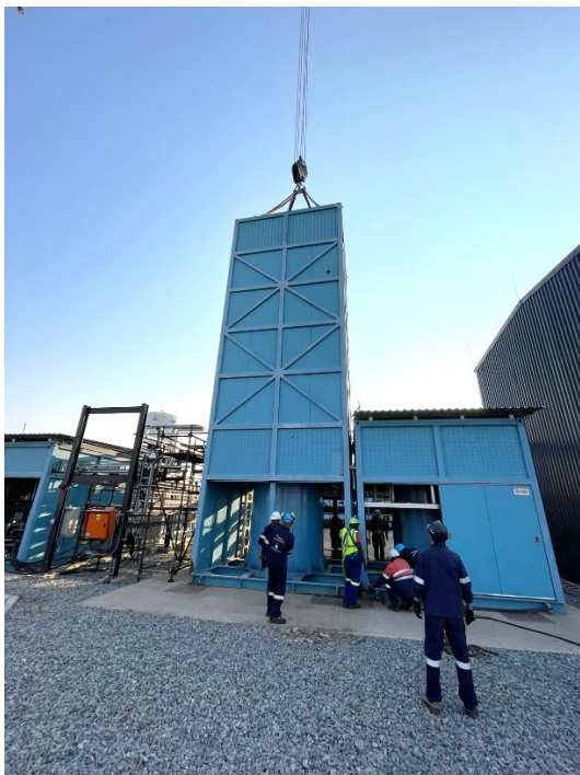
Figure 1: Cold box back in place at the Virginia Gas Project
