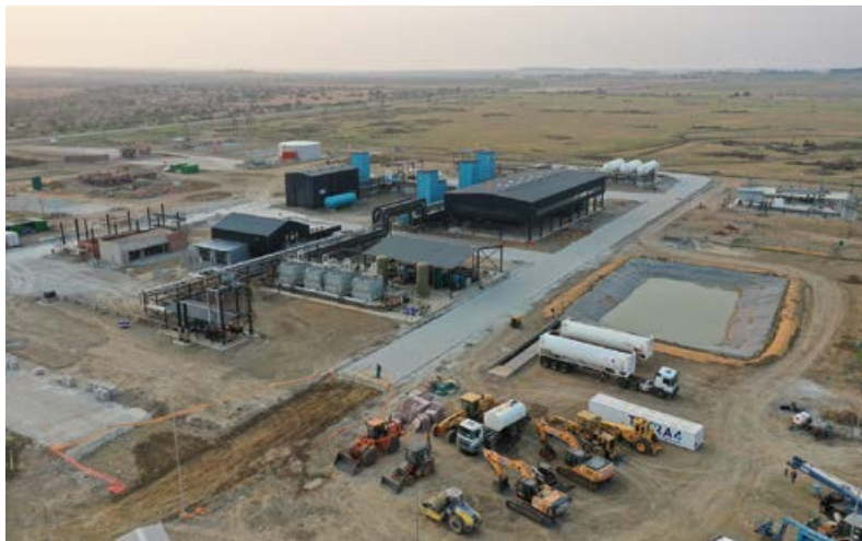
Virginia Gas project.
