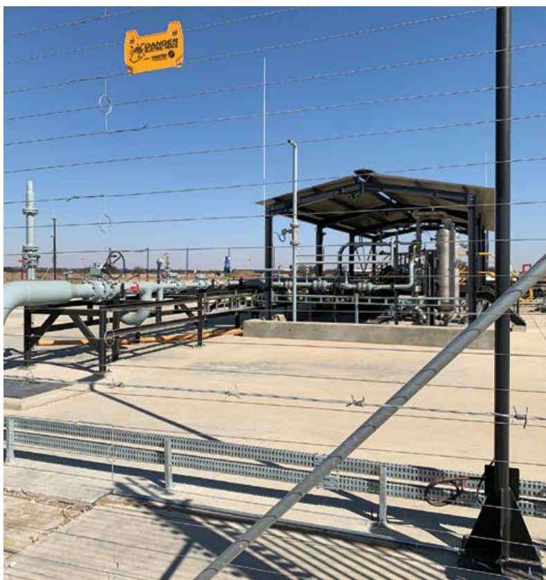
Virginia project compression station.
