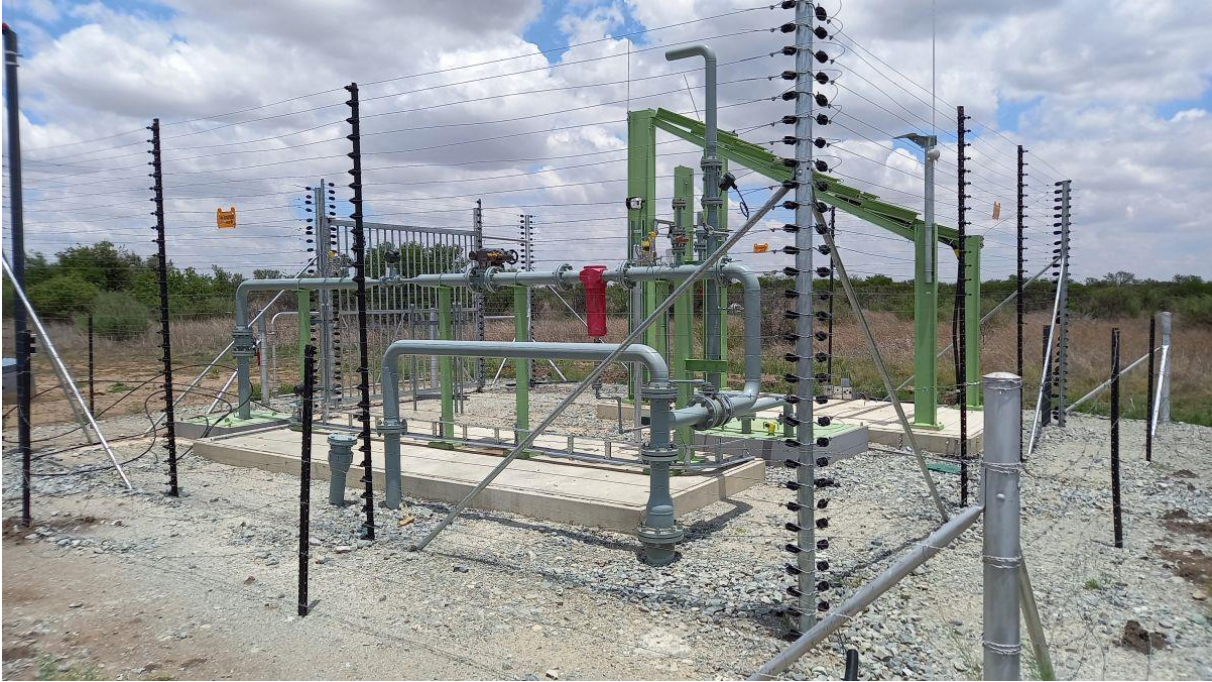
Figure 8: The production wells were temporarily disconnected from the gas gathering pipelines due to theft and vandalism of the instrumentation and cabling at the production wells.
