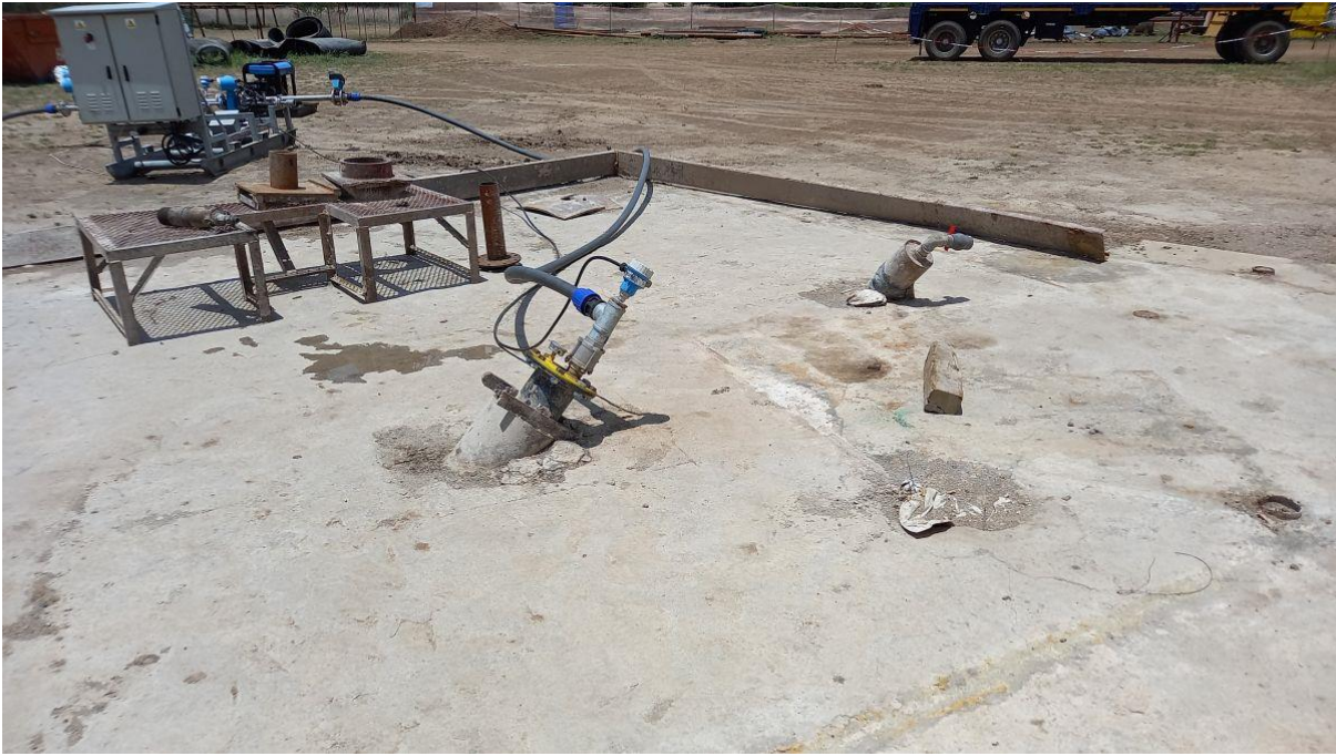
Figure 16: Drilling of the well R2D2 (b) was undergoing yield testing after drilling were completed.
