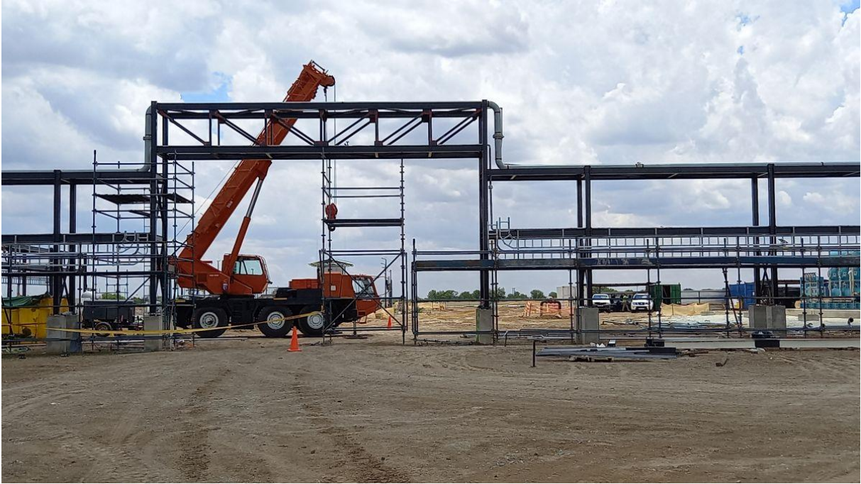
Figure 10: Installation of the pipelines and cable racks to the LNG storage tanks and loading bay continued.
