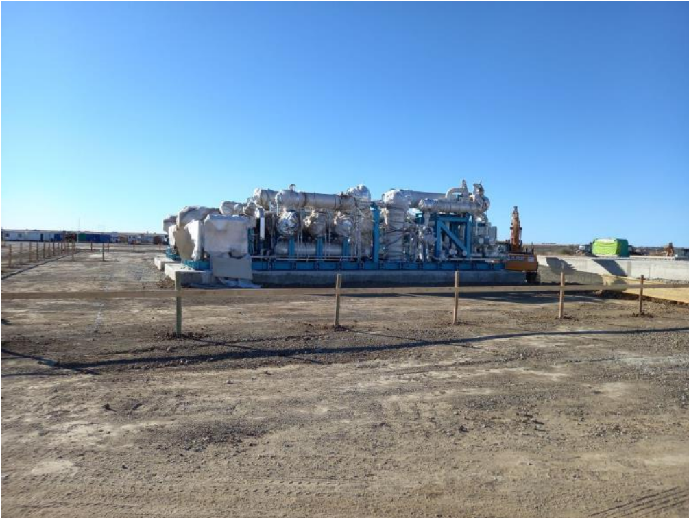
Figure 9: Main compressor units installed.
