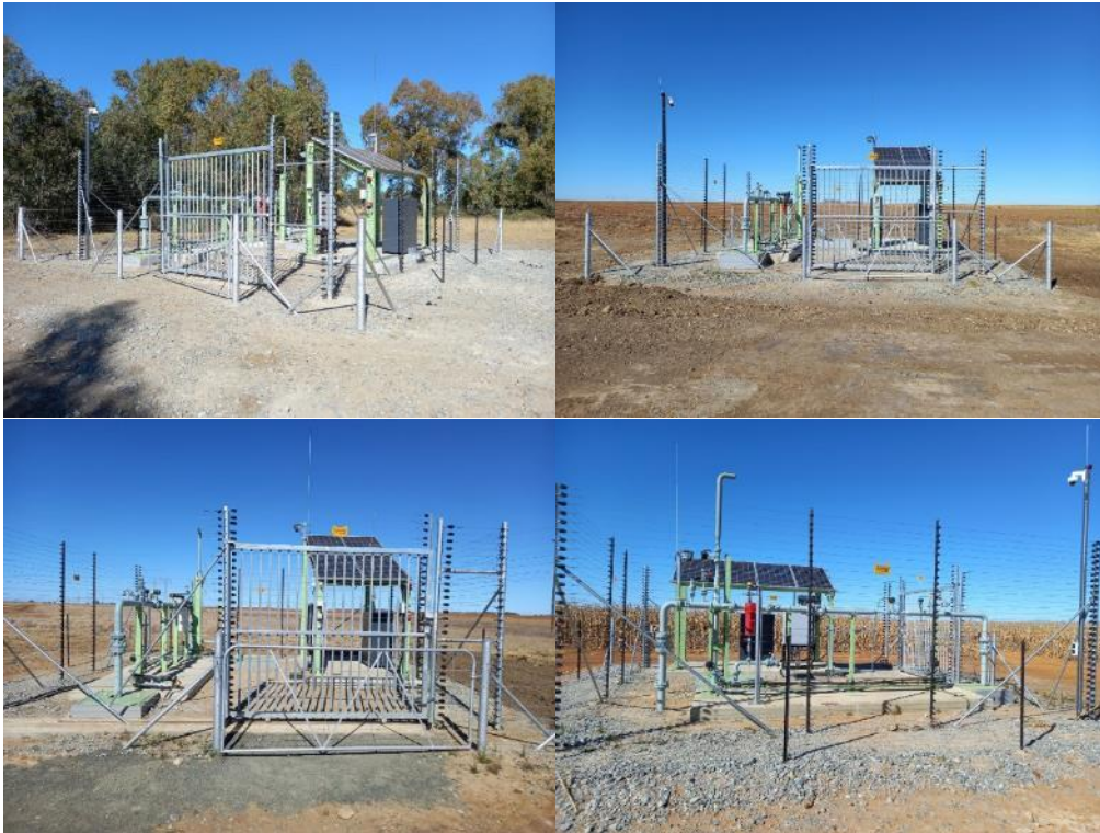
Figure 12: Installation of the Cluster 1 gas wells was mostly completed (EX01, 1400, ST23, DBE1).
