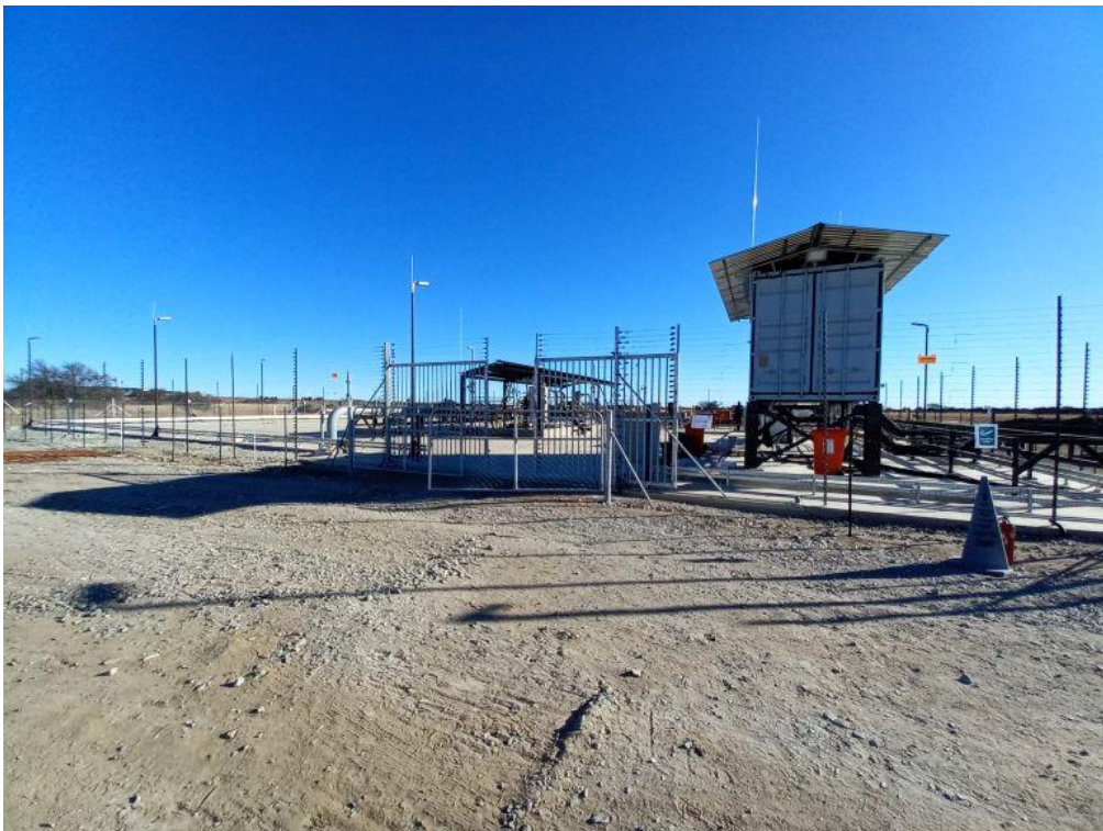
Figure 11: Installation of the compressor equipment at compressor Station B at the LNG/ Helium Plant was completed and commissioned.
