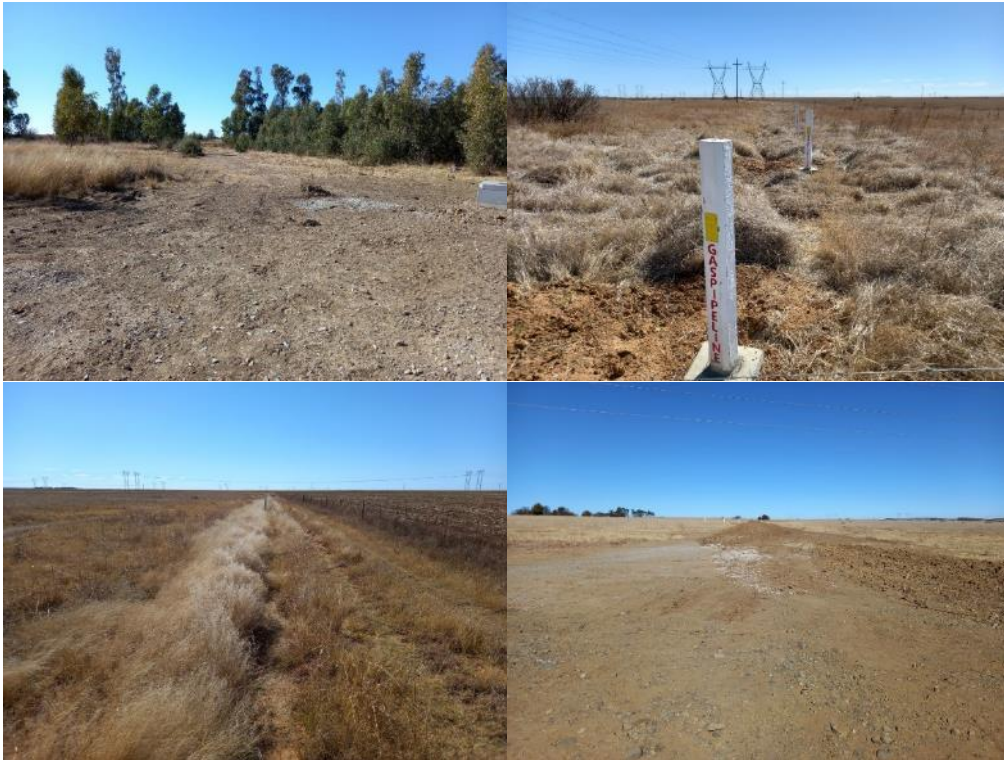
Figure 14: Rehabilitation of the pipeline was mostly completed with some punch items to be addressed.
