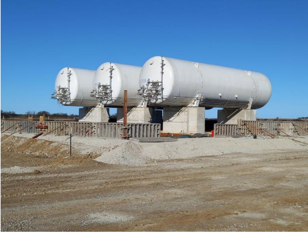
Figure 8: Concrete works for the construction of the bund wall around the LNG storage vessels.
