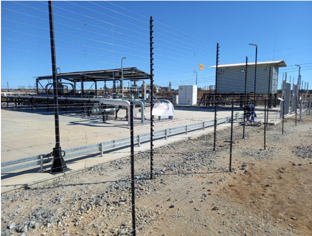
Figure 10: Installation of the compressor equipment at compressor Station A (ST23) was completed and commissioned.
