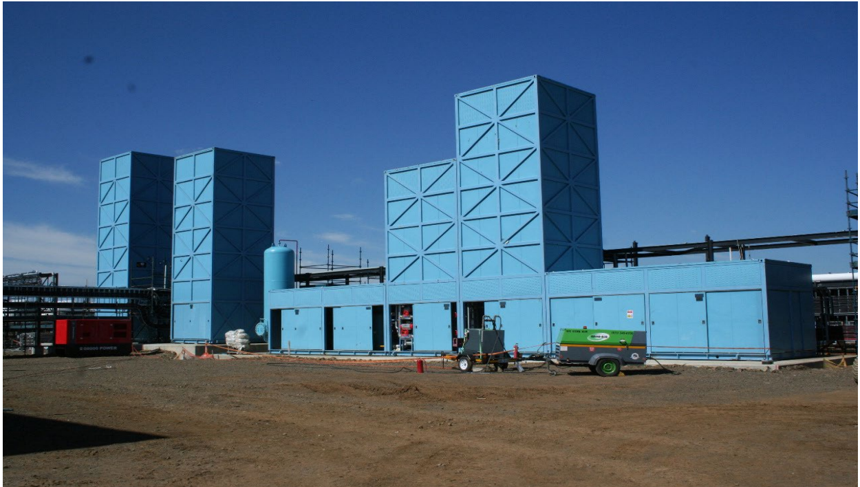
Figure 2: Front view of the gas pre-treatment and LNG cold boxes
