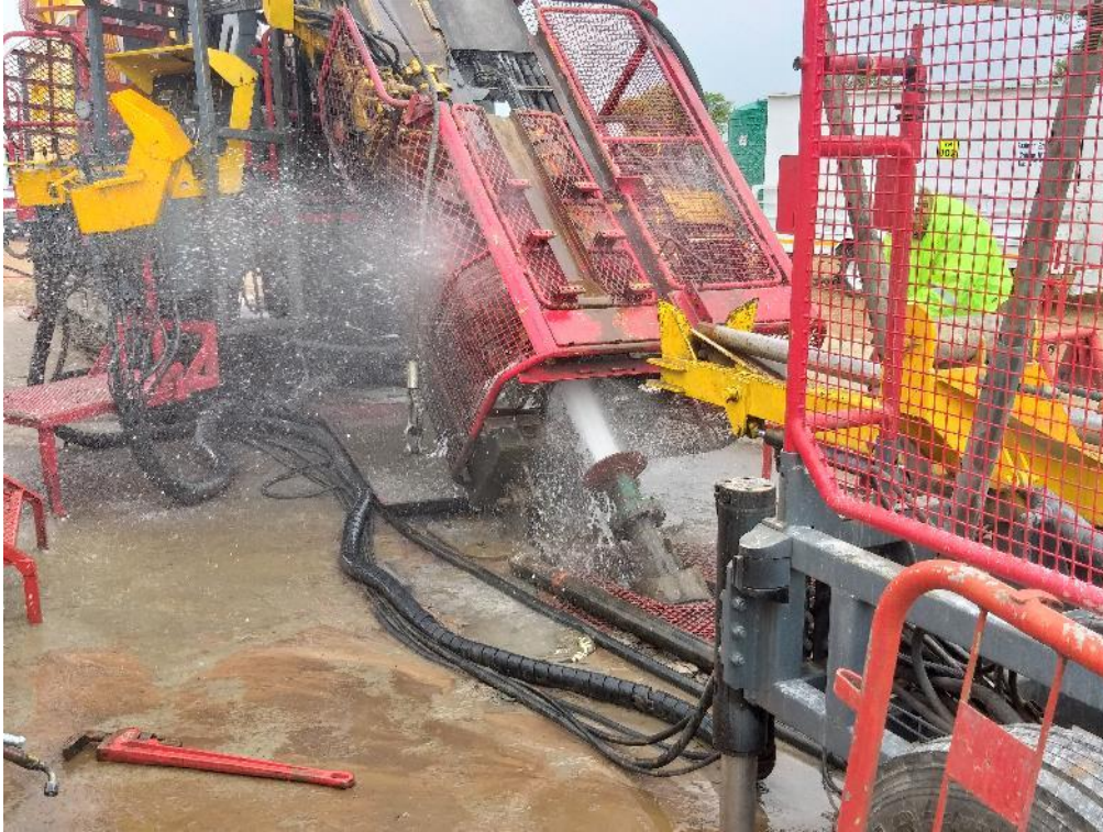
Figure 1: Drilling at the NEA02HT4 drill site continued at the time of the audit.
