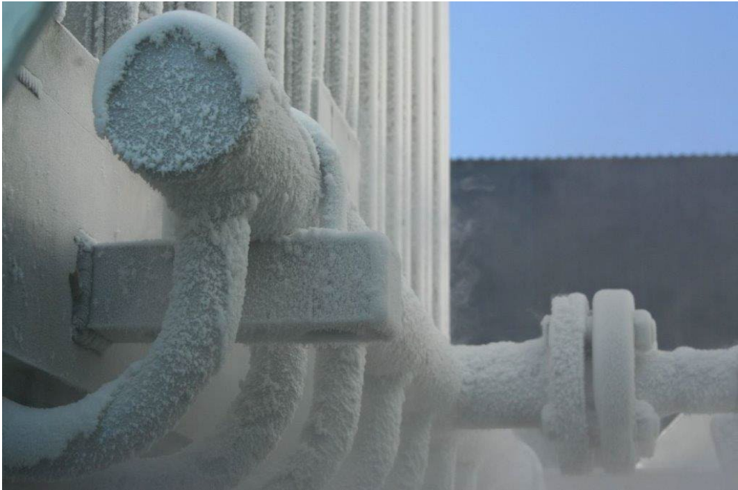
Figure 1: LNG Vaporiser being brought down to cryogenic temperatures, freezing water vapour in the air
