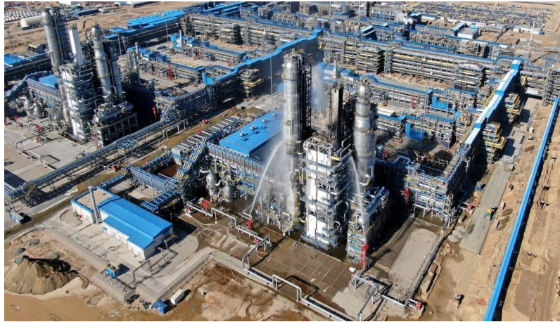
Exhibit 5 – The second train of the Amur gas processing plant following the fire that started on 8 October 2021
